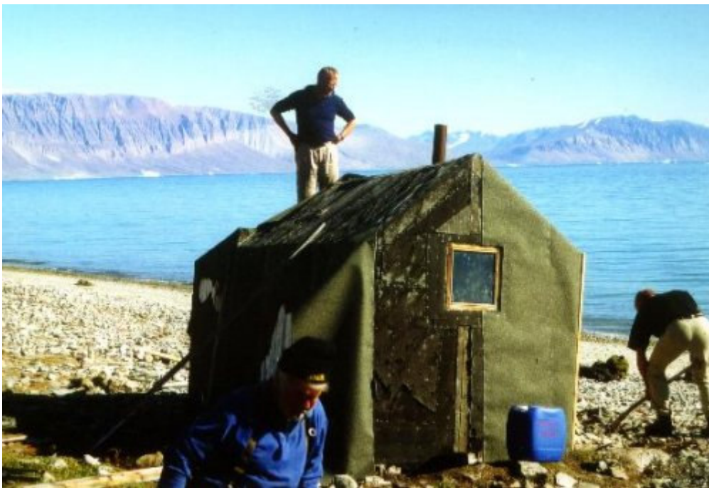
Persistent work was done attaching new felt, a new door was made and set in place and the window was repaired and a shutter fitted.
