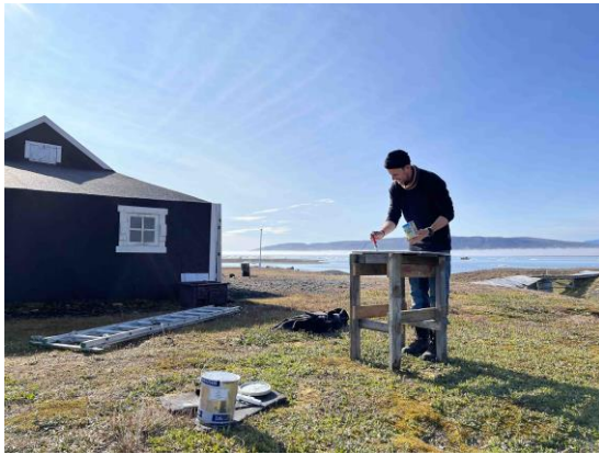
The woodwork needed painting, the gable antlers were loose and there was a lot of work with the roofing felt.
